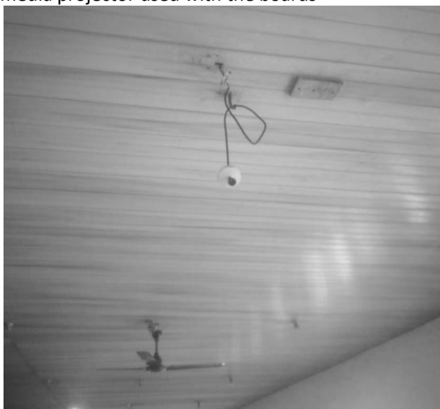
Fig. 3: Multimedia projector seating on the ceiling, after the projector was stolen
